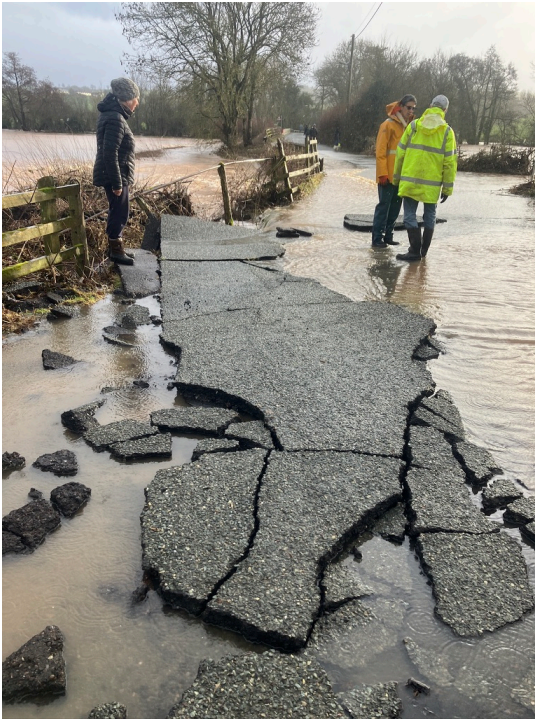
The damage to Station Road
