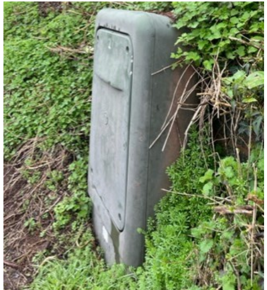
The rather older distribution box at Station Cross
