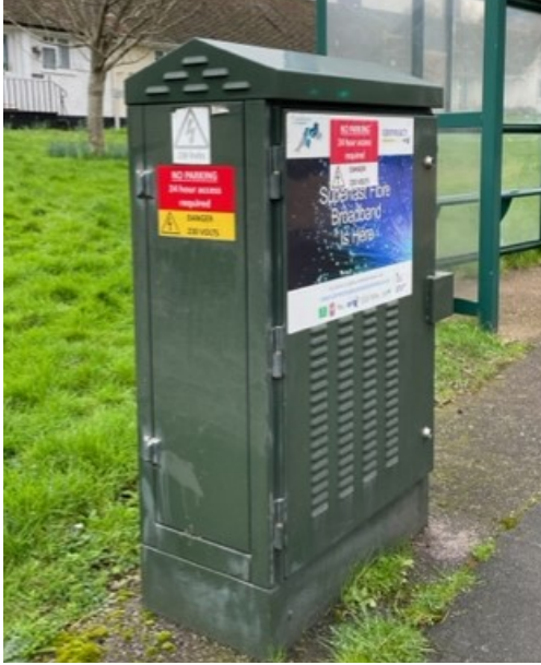
The fibre to the cabinet box on the green
